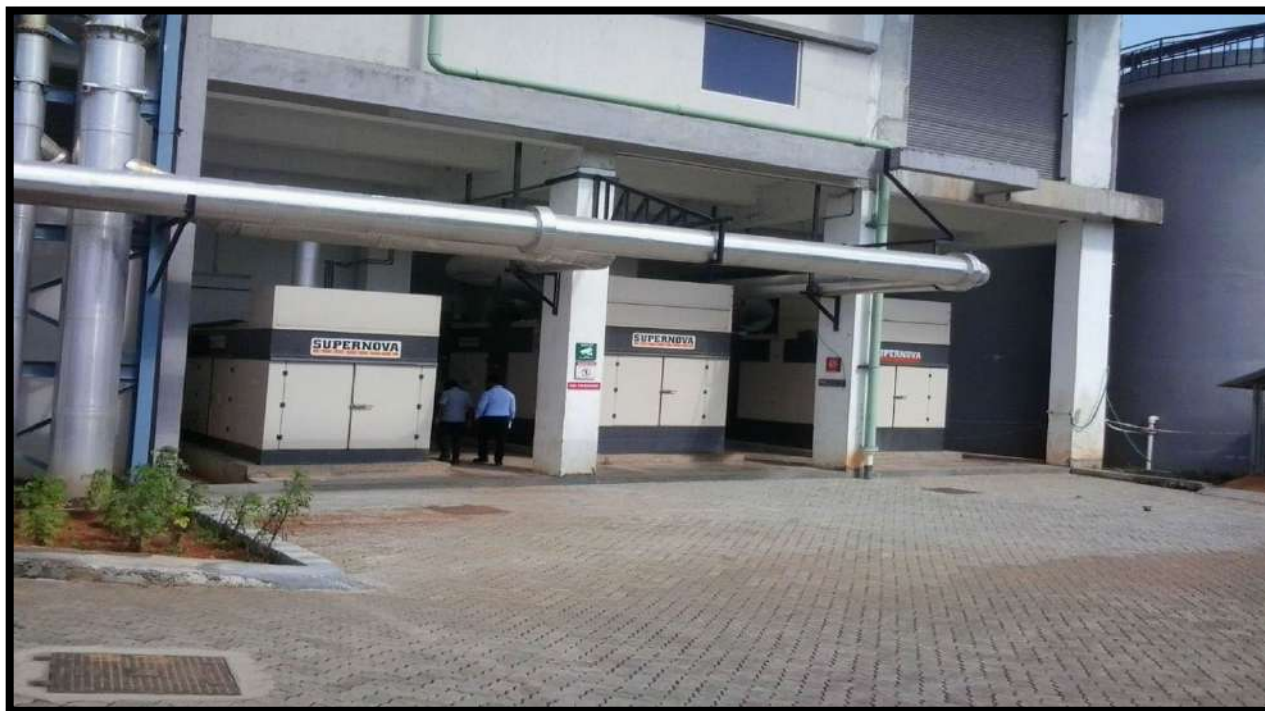
Photograph of DG stack
